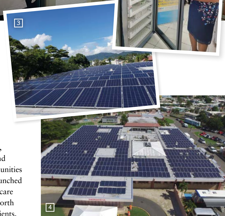
[3] [4] The Direct Relief-funded battery and solar power system at Family Health Center in Arroyo, Puerto Rico. (Courtesy photo)
